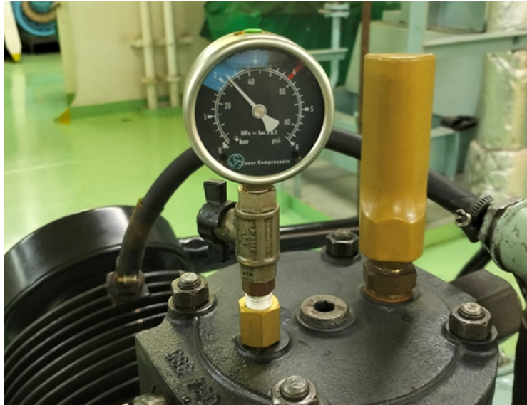
Gambar 3. Pressure Gauge 1st Stage
