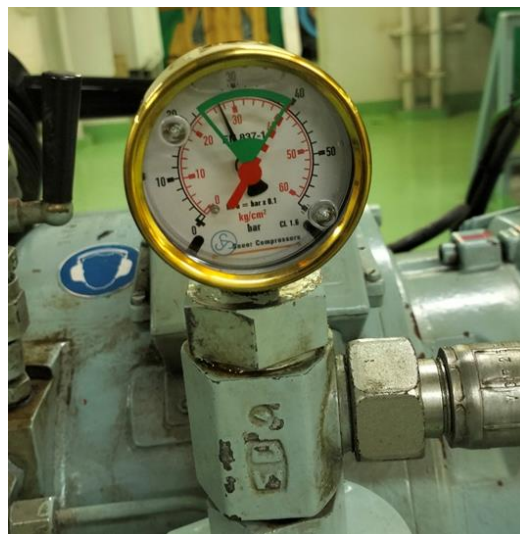
Gambar 5. Pressure Gauge 3rd Stage
