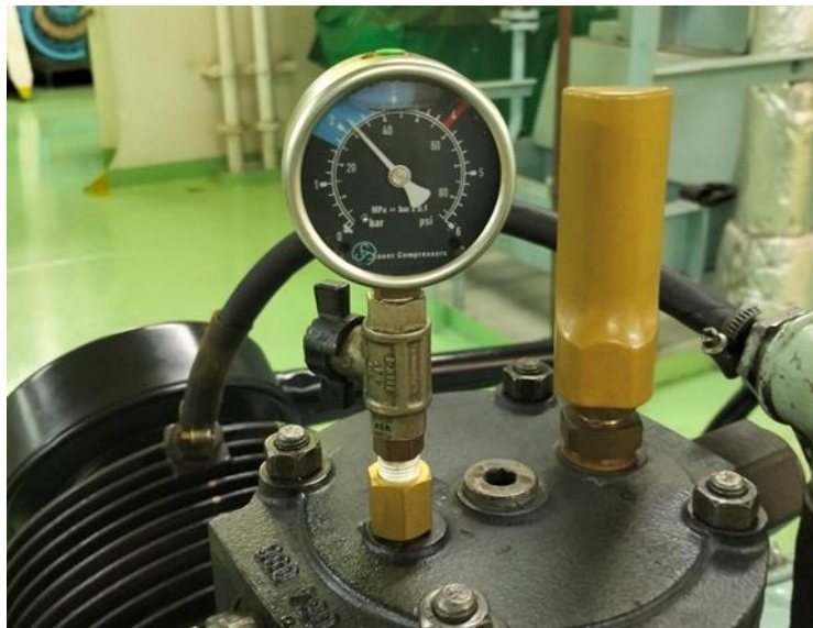
Gambar 3. Pressure Gauge 1st Stage
