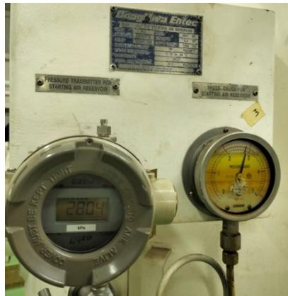
Gambar 6. Pressure Gauge Air Reservoir
